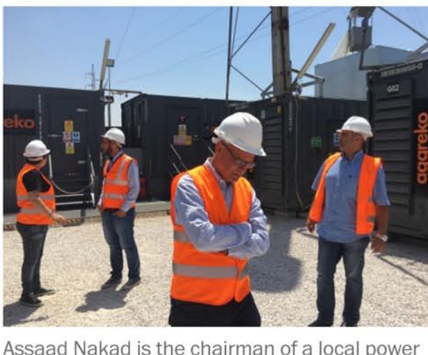
Assaad Nakad is the chairman of a local power company in Lebanon that provides round-the-clock electricity. He's touring a power plant that he recently had built for his home town of Zahle, Lebanon on Aug. 15, 2016. (Hugh Naylor/The Washington Post)
